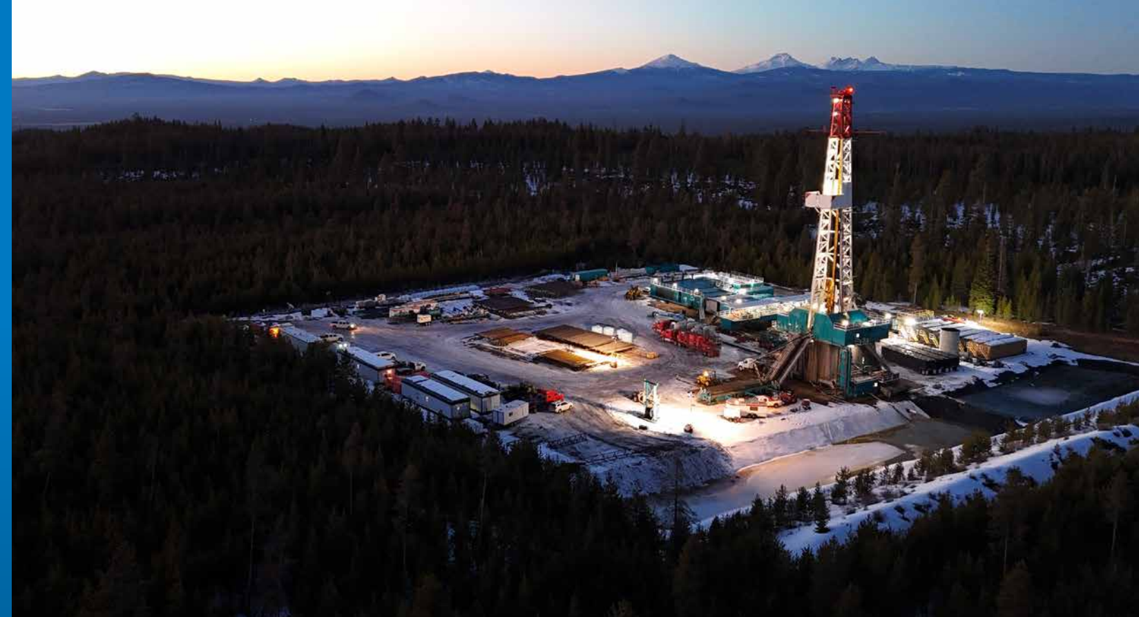
Photo from Mazama Energy
